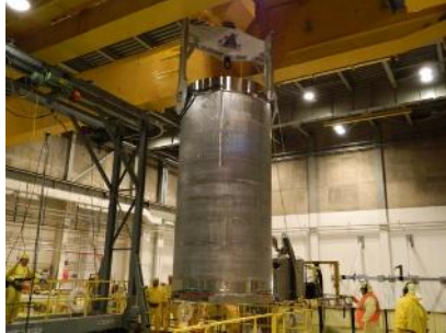
Transfer Cask Being Lowered into Spent Fuel Pool
